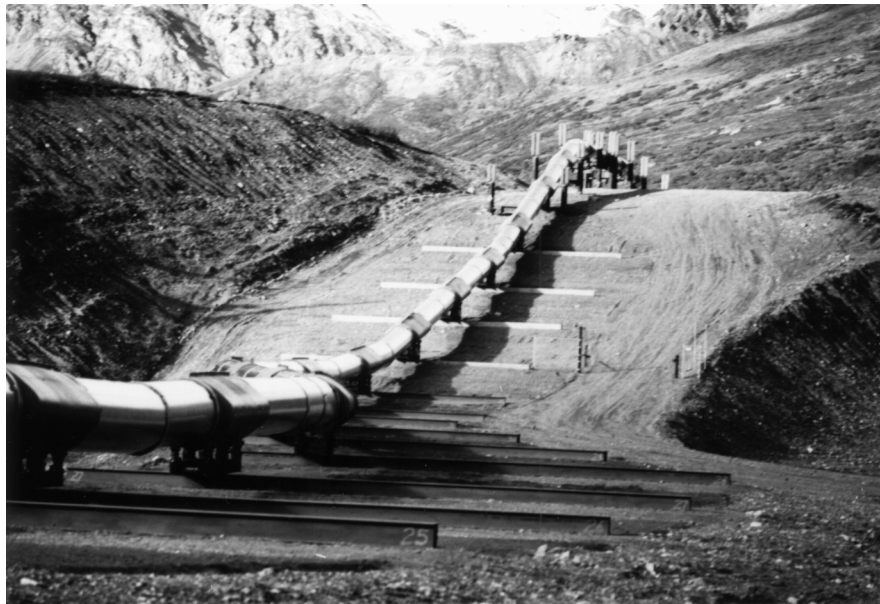
Figure 6. Special design of the Trans-Alaska pipeline to accommodate surface faulting at the Denali fault. The part of the pipeline in the background, beyond the active fault zone, is elevated and has the normal above-ground design. The part of the pipeline in the fault zone (foreground) is at ground level and rests on steel or concrete beams that allow the pipe to move horizontally and vertically. The design fault displacements are 6.1 m strike shift and 1.5 m dip shift. The pipe is 1.22 m (48 in) in diameter. Photograph by 0. J. Ferrians, Jr., U.S. Geological Survey, September 19, 1977.
