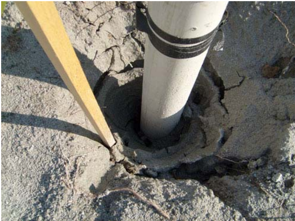
Figure 52. Grout collapsed around PVC pipe in a cross-hole tomography bore hole.
