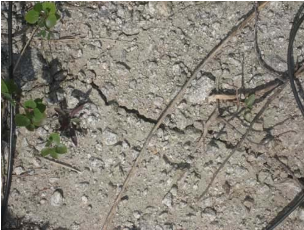
Figure 28. Crack from Shot 4 observed while walking around the borehole.
