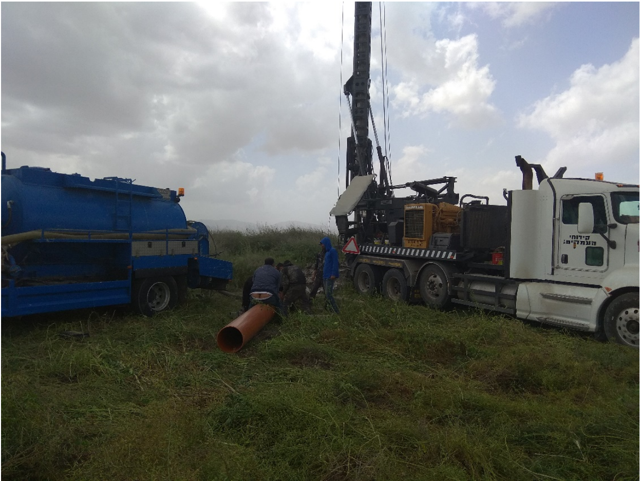
Figure 2 – Bucket auger drilling rig mounted on a truck, bentonite tanker and the plastic pipe, at borehole #12.
